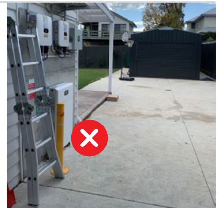
Figure 3.2: As noted in Figure 3.1, there is adequate area for a car to drive beyond the edge of the battery, this requires additional mechanical protection be installed on the trailing edge of the battery.
