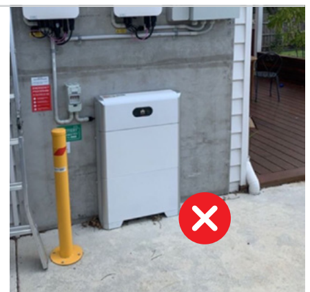
Figure 3.3: The absence of trailing edge protection in an area accessible by vehicles makes this system non-compliant.
