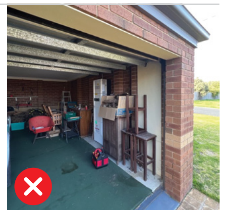
Figure 1.3: A vehicle could enter into this space, meaning that fixed vehicle mechanical protection would be required regardless of any non-fixed objects that could be installed.
