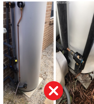
Figures 3 and 4: Although an attempt to angle this drain termination point away, it is directed towards electrical equipment which could cause splashing of water or steam to enter the electrical terminal cover.
