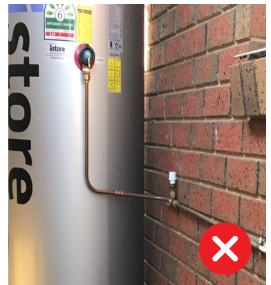
Figure 5: The drain has been installed with an overflow relief which could force hot water horizontally at height if the drain downstream becomes blocked.
