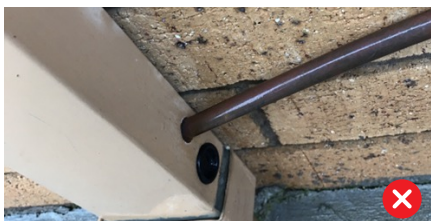
Figure 4: This drain is discharging into the downpipe but may not be readily discernible in the event there is an issue with the TPR valve or hot water system. It may also become blocked by a blockage or surcharge in the stormwater drainage system.
