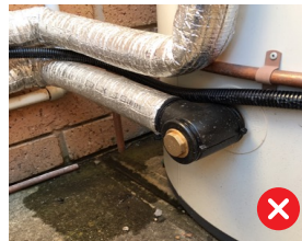
Figure 2: The angle and vicinity of this drain termination point, along with the path graded back to the structure wall, may affect the slab and foundations in reactive soils.
