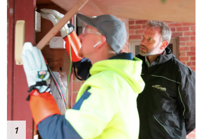
1. Testing the earth continuity back the main earth bar, while wearing PPE (testing).
